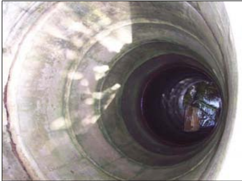
Figure 38: A well contaminated by garbage.
